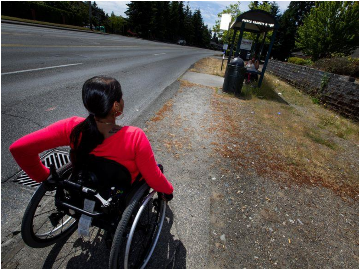
Krystal Monteros, chair of the Tacoma Area Commission on Disabilities, shows where a sidewalk to a Tacoma bus stop becomes a stretch of gravel. (Ken Lambert / The Seattle Times)
