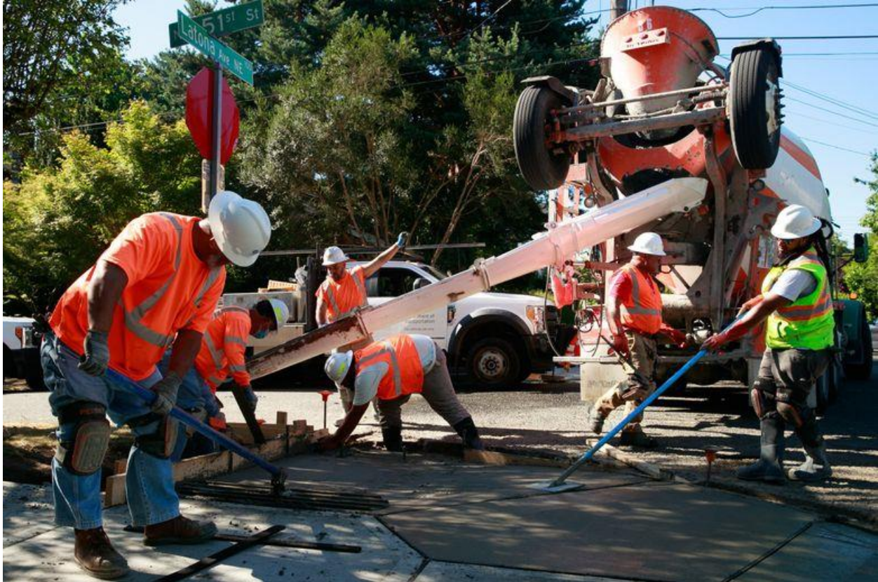
1 of 3 | Seattle Department of Transportation crews, including Pita Moimoi, left, work on improving the accessibility of sidewalks at Latona Avenue Northeast and Northeast 51st Street in Seattle in late July. (Erika Schultz / The Seattle Times)
