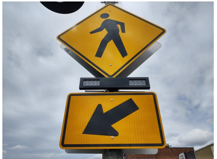
Signs with a rectangular rapid flash beacon (RRFB) mounted on a light pole at 1st Avenue and Main Street (April 24, 2020).
