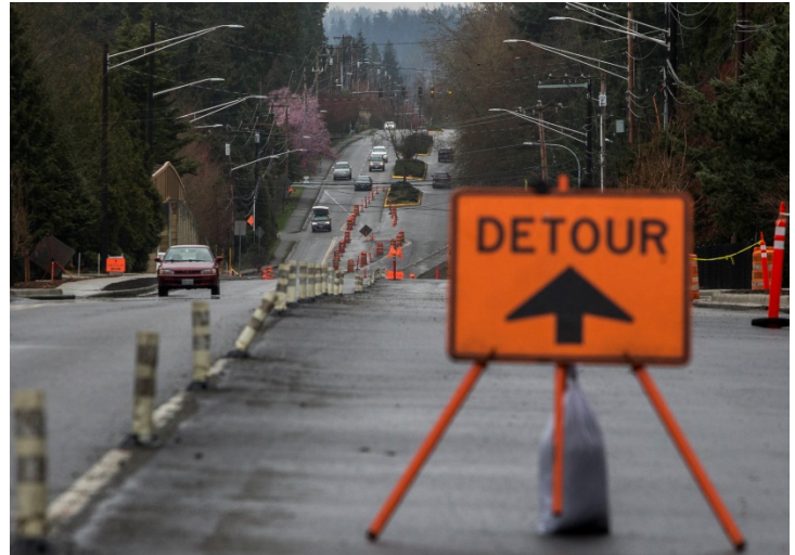
Cars merge and navigate the construction along 36th Avenue West on March 13 in Lynnwood. The road project is nearing completion. (Olivia Vanni / The Herald)
