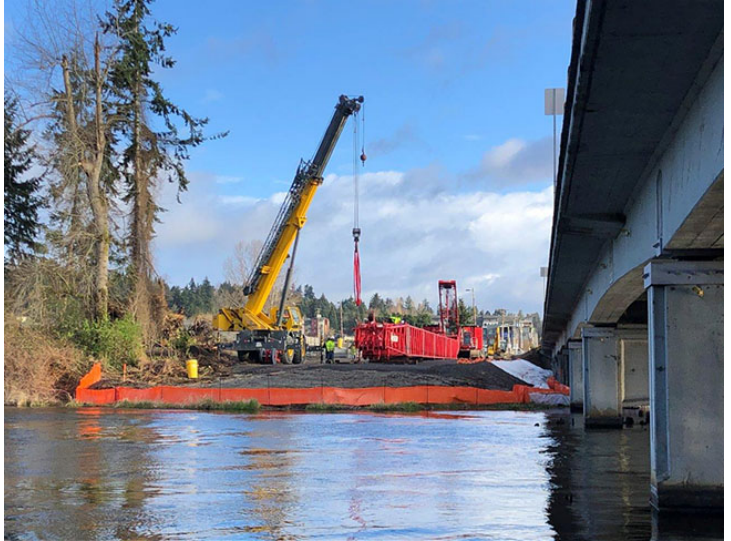
Workers are building a berm and landing area for a crawler crane. Photo courtesy of the City of Kenmore
