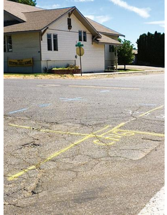
ROADWAY INSTRUCTIONS — The colorful chalk markings are street locator marks for the water main replacement crew to follow during the mid-July water main improvement project in Granger.
