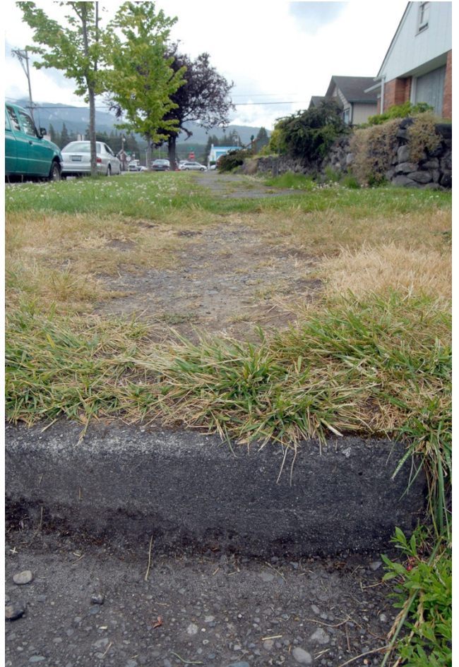
A curb without a wheelchair access cut stands at the corner of Francis and Georgiana streets in Port Angeles.
