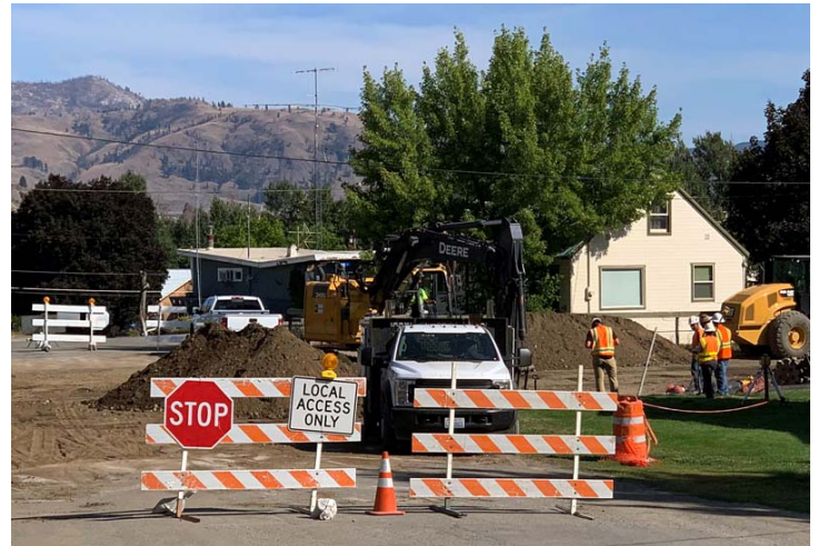
A crew from Hurst Construction excavated Canyon Street at Fifth Avenue in Twisp on Aug. 28. The Canyon Street project was scheduled to be completed by Aug. 26, according to town officials. The town has informed Hurst that it will seek approximately $2,000 per day in damages to compensate the town for any additional costs.
