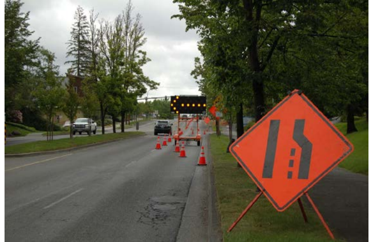
Traffic goes down to one lane when heading east along Harbour Pointe Boulevard Southwest towards Mukilteo Speedway due to construction of the Harbour Pointe Boulevard Southwest Widening Project. The project will cause delays and lane closures through this fall. Construction started recently.
