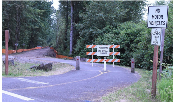
Enumclaw’s expansion of the Foothills Trail is already underway, and is planned to be finished by fall 2019. File photo
