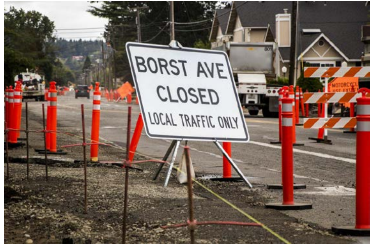
The Borst Avenue Project closes the road to local traffic only as crews remove sections of sidewalk and blacktop, Friday morning in Centralia.
