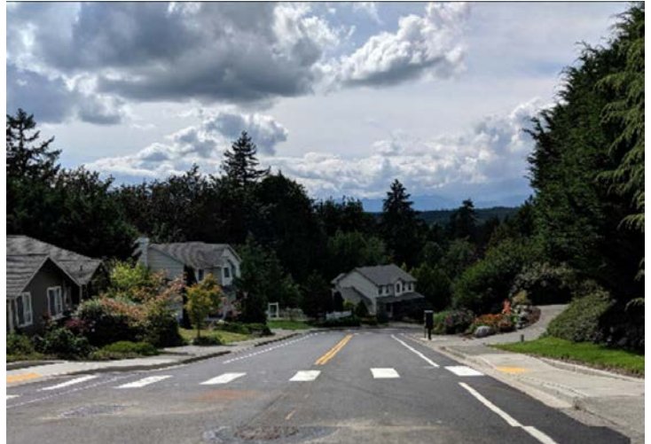
Newly painted fog lines ad a finishing touch to the road improvements.
