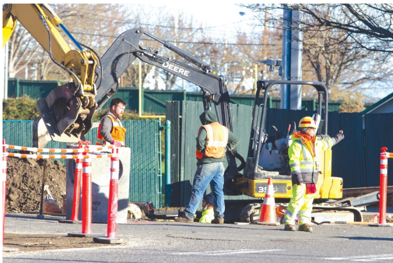
A construction crew works on the Jefferson Street sidewalk extension project at the northeast corner of Quincy and Washington streets. The $650,000 project was expected to be completed by the end of 2018.
