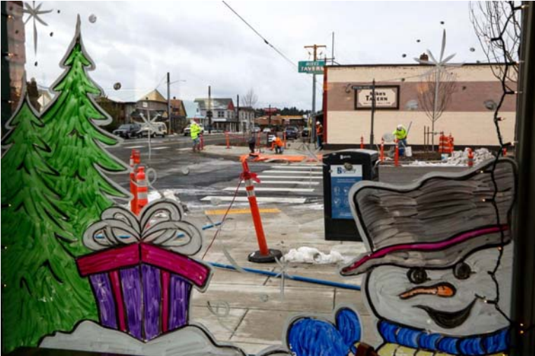
Orange caution cones and construction workers dot the sidewalk in downtown Cle Elum as concrete is poured and spread to form new sidewalks on Friday. The sidewalks are part of a Cle Elum downtown revitalization project.
