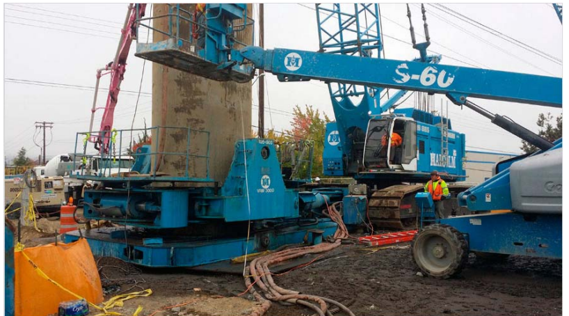
Crews will install shafts like this next year to help support a new overpass along South 228th Street over the Union Pacific Railroad tracks. COURTESY PHOTO, City of Kent
