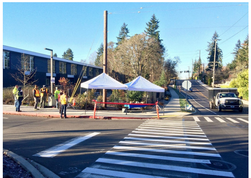
As part of the project, concrete curbs, sidewalks and bicycle lanes were constructed on both sides of Southeast 40th Street, from Island Crest Way to Gallagher Hill Road. Photo via Facebook
