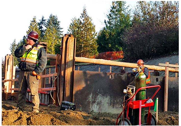
Work has resumed on the Tremont Street widening project. (City of Port Orchard photo)
