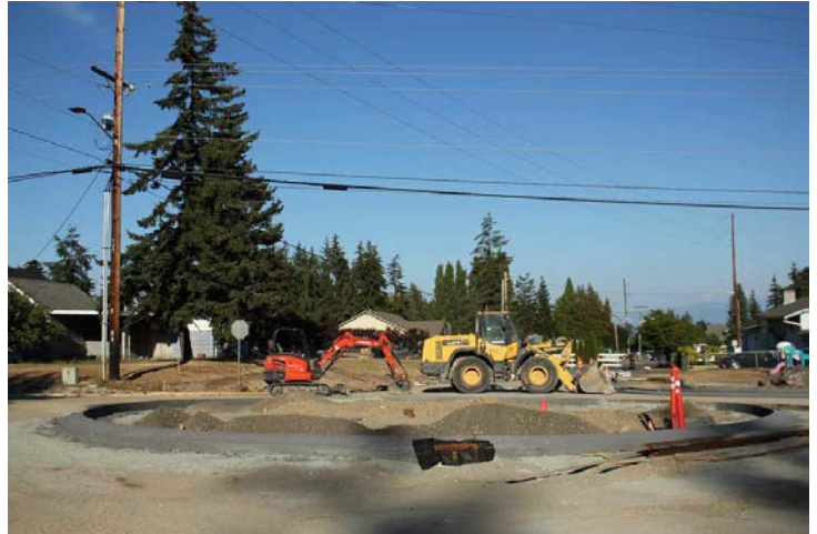
Completion of a new roundabout at 32nd Street and D Avenue was delayed due to a strike. Here, the roundabout is seen on Aug. 27.
