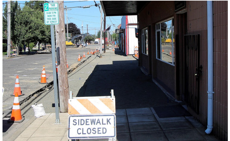
A look east along Marcy Avenue in Montesano taken July 16. Two blocks between South Main and River Street South have long been a maintenance headache for city street crews and are getting a complete rebuild over the next month or so. DAN HAMMOCK | TWIN HARBORS NEWSPAPER GROUP
