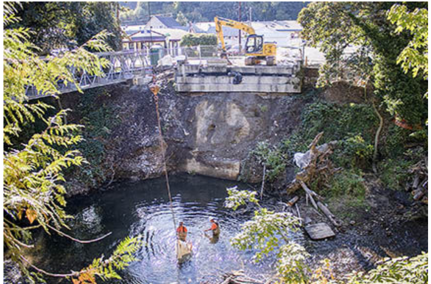
Two construction workers wade through the water, one holding a large construction bag attached to a crane, at the Fir Street Bridge construction site in October, 2017 in Winlock. Jared Wenzelburger / jwenzelburger@chronline.com )
