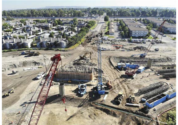
Construction crews work on the Duportail Bridge on the north side of the Yakima River in Richland. The estimated $38 million project will link Richland's waterfront, central business district and Queensgate areas. Watch a video at: tricityherald.com/video Bob Brawdy Tri-City Herald
