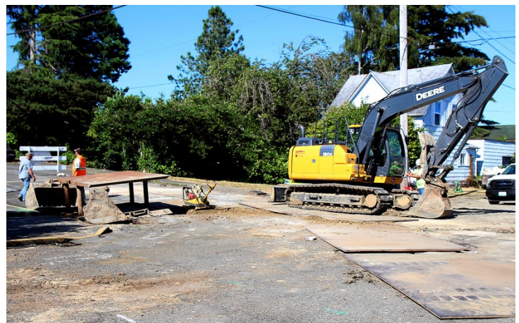
The intersection of Marcy Avenue and South River Street in Montesano is now covered in steel plates as contractors begin a complete rebuild of Marcy Avenue between South Main and South River. DAN HAMMOCK | TWIN HARBORS NEWSPAPER GROUP
