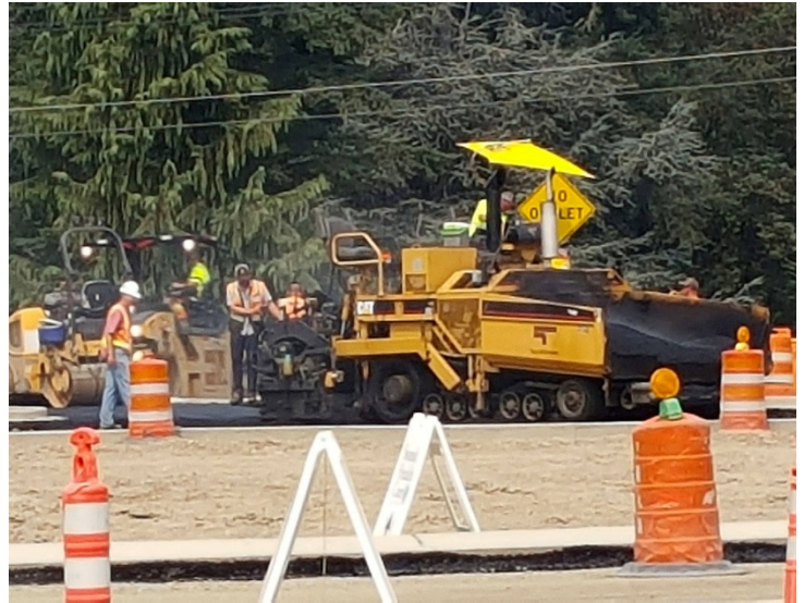
Construction crews work on the Tremont Street widening project prior to a three-week strike that ended Sept. 6. (Bob Smith | Kitsap Daily News file photo)
