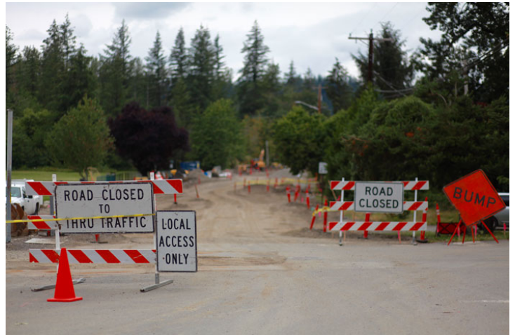
Construction began on First Street in Sultan around the start of June, and is expected to continue through the end of October. A short stretch of Eighth Street will also be repaved this season.
