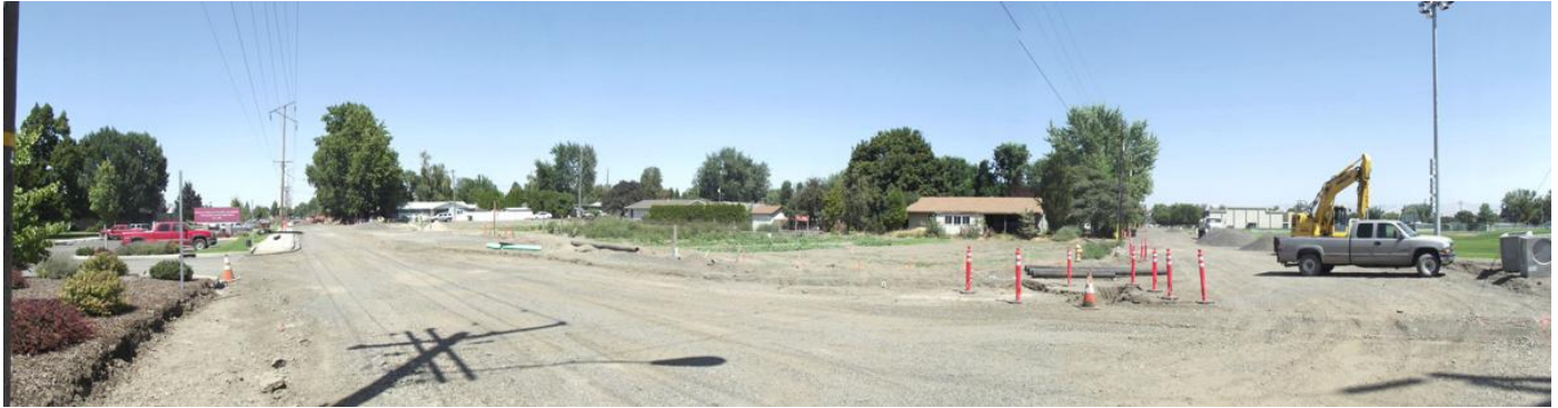
Academy Way and the West end of Fourth Street in College Place are being redone. Brenden Koch
