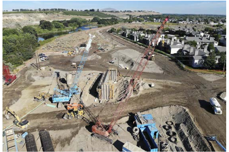
Crews work on the future Duportail Bridge on the north side of the Yakima River in Richland. The estimated $38 million project will link Richland's waterfront, central business district and Queensgate areas. Watch a video at: tricityherald.com/video Bob Brawdy Tri-City Herald
