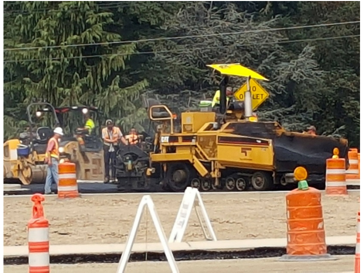
Work on the City of Port Orchard's Tremont street widening project has been halted because of a contract dispute by union equipment operators.
