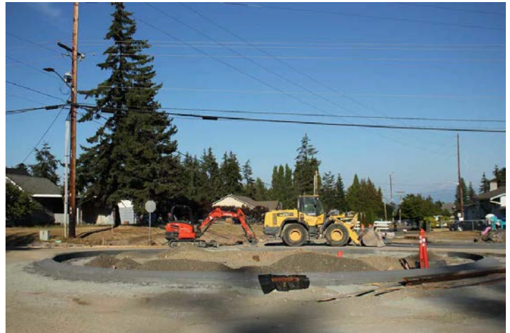
Completion of a new roundabout at 32nd Street and D Avenue was delayed due to a strike. Here, the roundabout is seen on Aug. 27.
