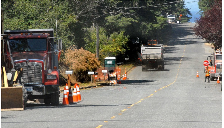
A dump truck makes its way through a construction zone as flaggers control traffic along West 10th Street in Port Angeles on Wednesday. (Keith Thorpe/Peninsula Daily News)
