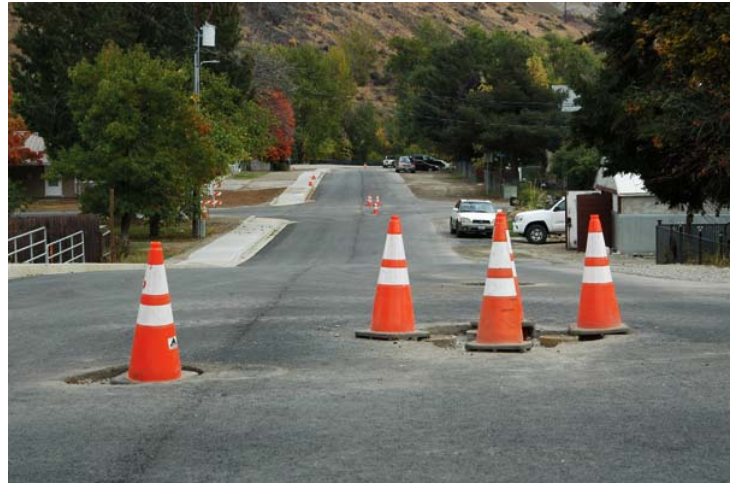
Newly paved streets, with new water lines beneath, are getting the finishing touches put on as a three-month-long project wraps up in Twisp.
