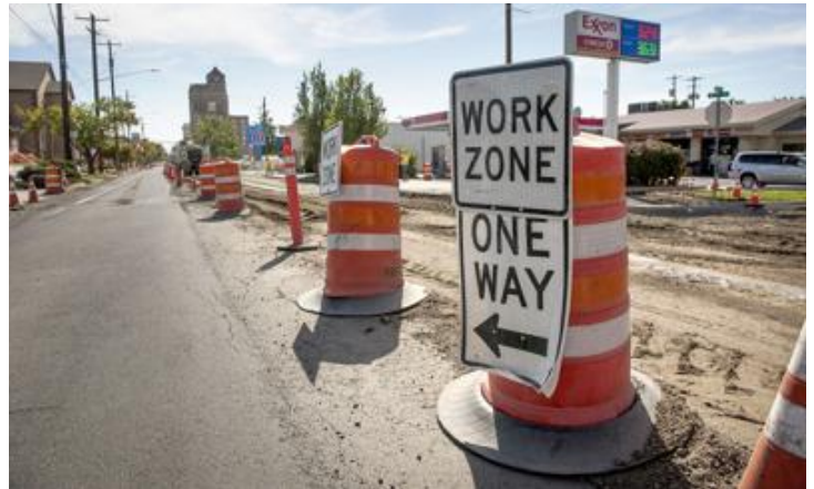
Work progresses on North Second Avenue in Walla Walla, in late September.
