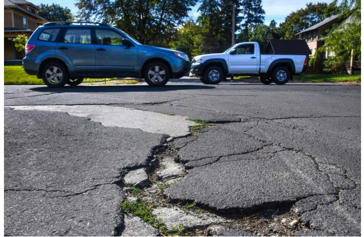
Vehicles travel over broken pavement on 14th Avenue at Madison Street on Friday in Spokane. (Dan Pelle / The Spokesman-Review)
