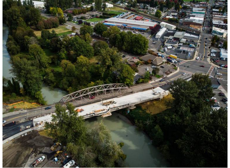
Construction crews work on the new Bridge Street bridge in Sumner on Wednesday, Oct. 3, 2018. Starting Oct. 8, traffic will be redirected onto the new bridge.
