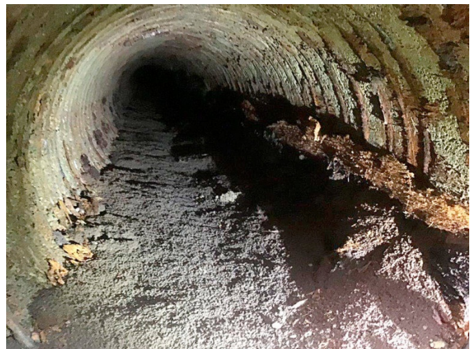
The Rucker Renewal utilities and road project ended up almost $2 million over the original budget because crews found unexpected conditions, including a void from deteriorated wood water pipes that had to be removed and filled. (City of Everett)
