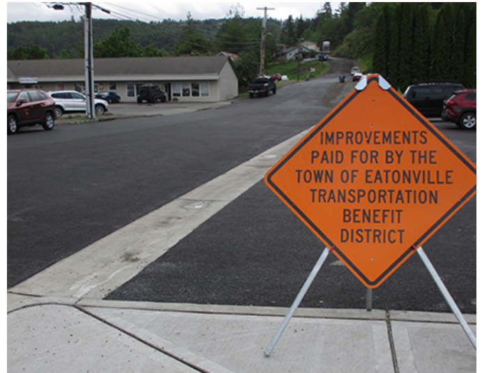
Photo courtesy of the Town of Eatonville: Not everything in 2020 was negative in Eatonville. The town was able to complete significant road projects, including one on Rainer Avenue South, using Transportation Improvement Board grant funds.
