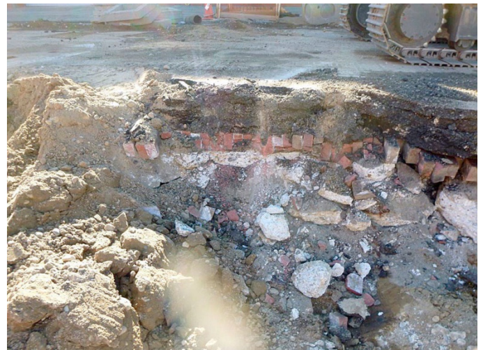
The Rucker Renewal utilities and road project ended up almost $2 million over the original budget because crews found unexpected conditions, such as this pavement-brick-pavement layering. (City of Everett)
